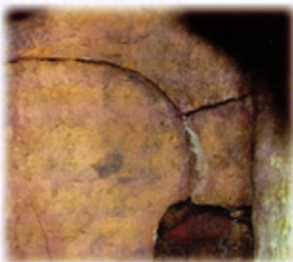
Damaged flue: Notice the moisture and the missing piece of flue tile.
