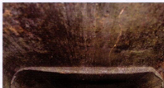
A crack like this can allow deadly gases to leak into the home, and can open the way for a chimney fire to turn into a house fire
